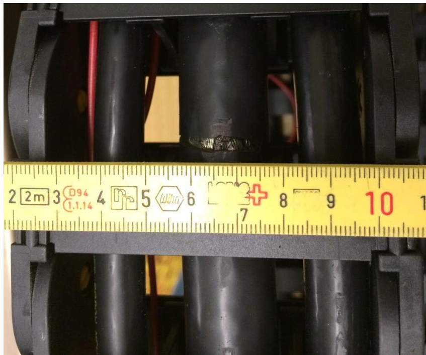
Figure 2 crack on cable sheath of 16(2 \times 1.5) \text{ mm}^2 , bending radius 160 mm
